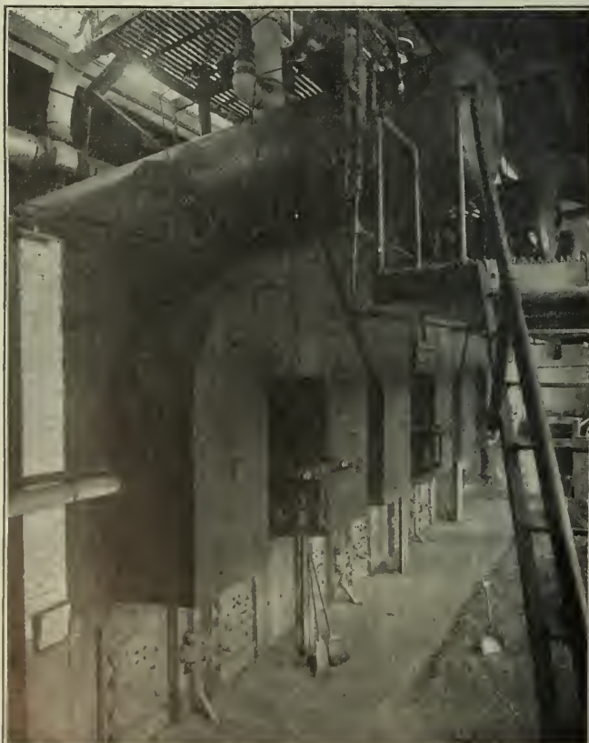
BOILER FRONTS AFTER CHANGE
